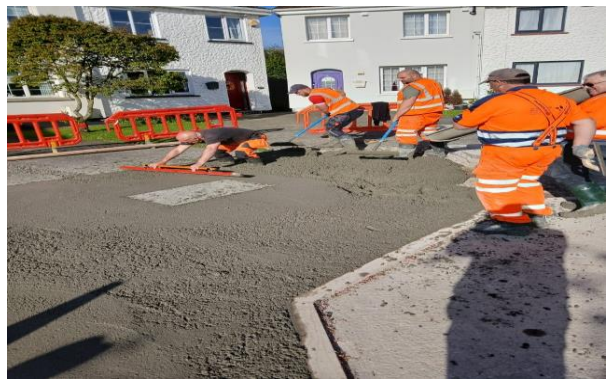
Footpath replacement works by Balbriggan Construction crew at Clonard Court as part of roads general maintenance programme.
