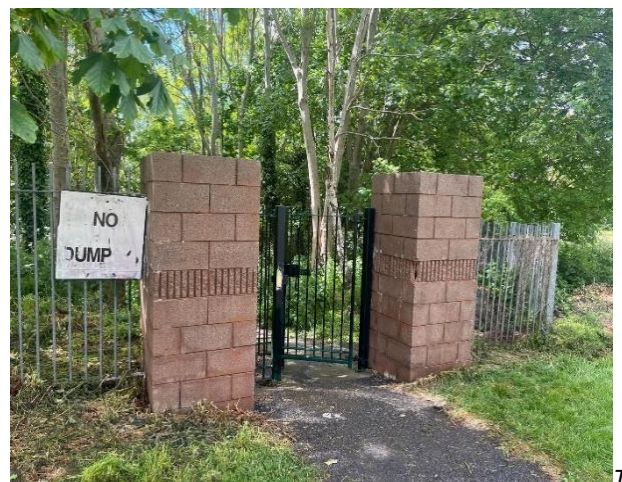
The piers leading into Tolka valley from Brookhaven Drive have been cleaned.
