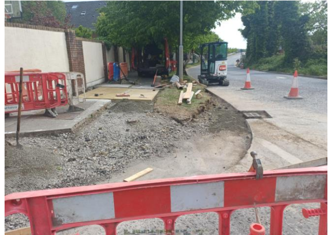
Junction Upgrade of Drynam Hall/Kettles Lane entrance. Entrance was narrowed with new tactile pavement and entrance ramp.
