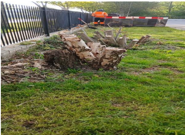
Stumps removed and ground reinstated with soil and grass seed in Damastown football Grounds and on Auburn Avenue.
