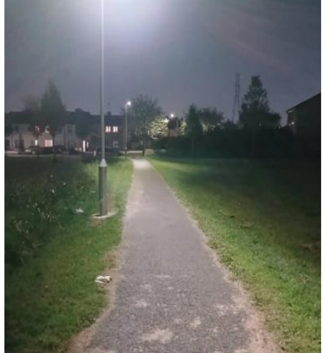
New Lighting Scheme on Whitestown Park Walkway, Coolmine
