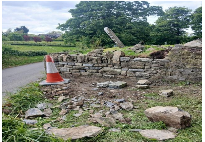
Repair of masonry brick wall at Oldtown by Construction crew as part of general maintenance works programme.
