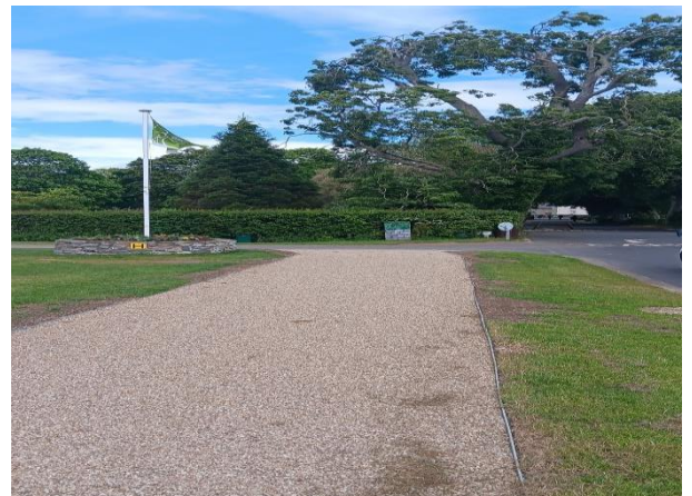
Top layer of Ballylusk stone laid on new path along the Vehicle entrance to Malahide Castle.
