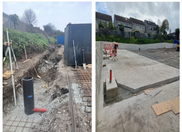
Works ongoing in Fancourt Depot for the construction of new EV charging points for electric fleet vehicles.
