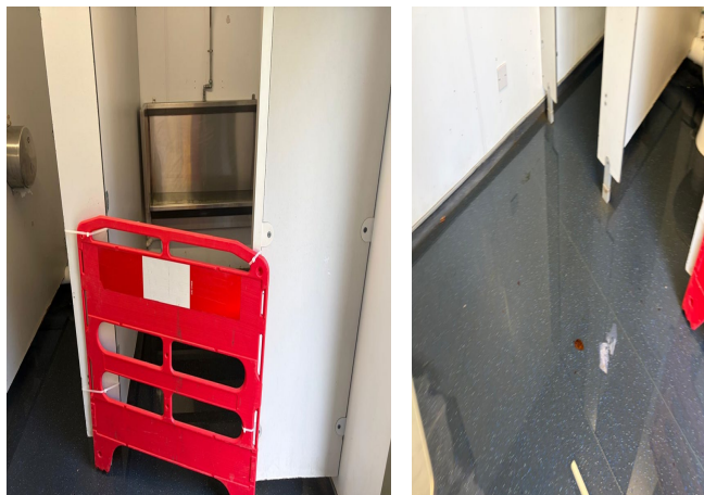
Area barriered off as the toilet and urinals were vandalised causing a leak/flooding on floor.
