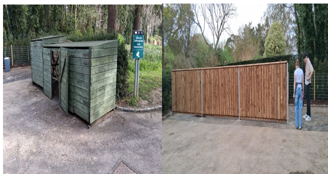
The old bin covers were removed and replaced with a more accessible & tidy solution at the back of the Avoca kitchen.
