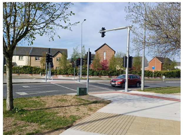
New signalised pedestrian crossing completed on the Ongar Distributor Road at Station roundabout.
