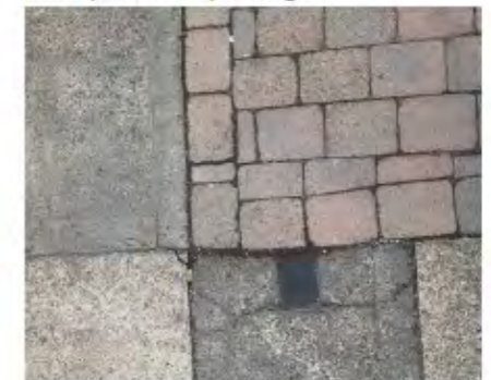
Poor and inconsistent paving materials
