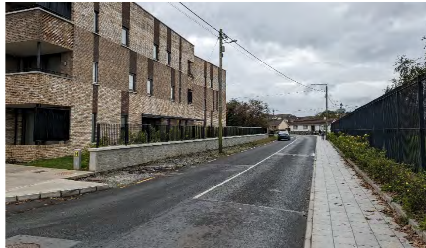
Fig. 9-1: Poor Quality Paving on Turvey Avenue
