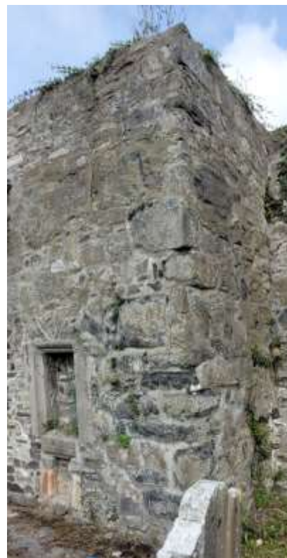
Vertical cracks to the east side of South elevation.
