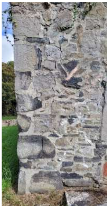
Vertical cracks to west side of south elevation.
