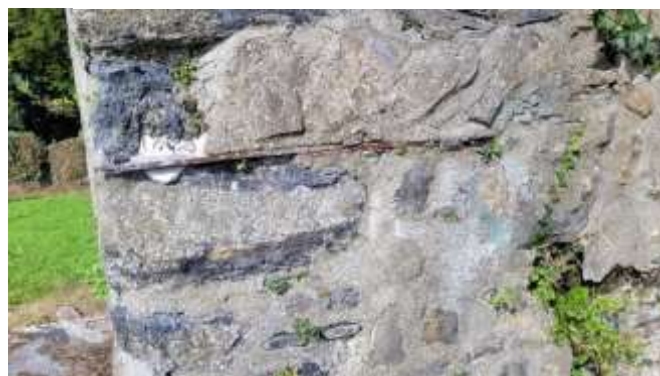
Corroding steel or wrought iron plate embedded in wall.
