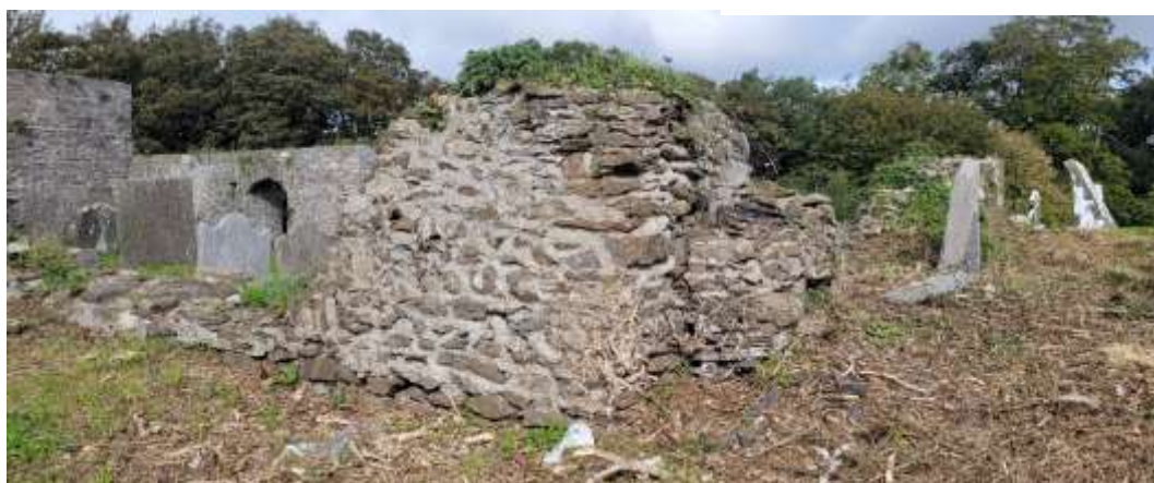
Poorly conceived repairs to southeast corner. Note buttressing stonework to right hand side in fragile condition.
