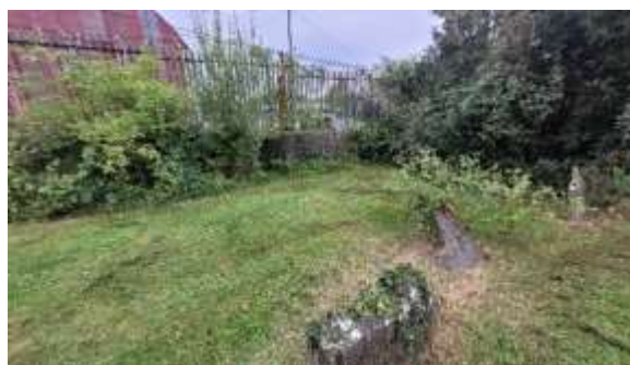
East and South walls are low rise masonry with palisade above. much overgrown
