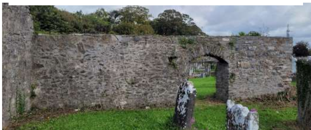
West end of north wall of nave in relatively stable condition.
