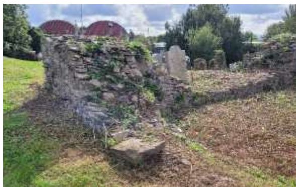
Northeast corner of nave in urgent need of stabilisation.
