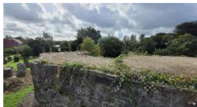
South side of tower top, flaunching generally intact and to outward falls but cracks + edges need attention.
