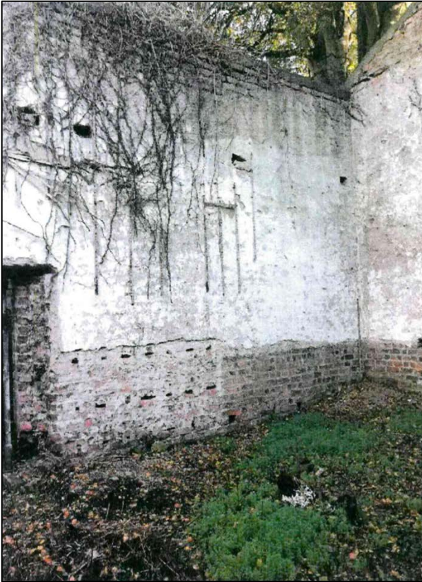
Plate 13: Vegetation growing on north internal elevation.
