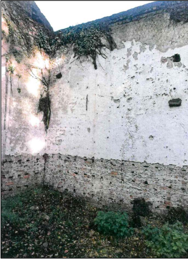
Plate 11: Vertical cracking at northwest internal corner of north elevation.
