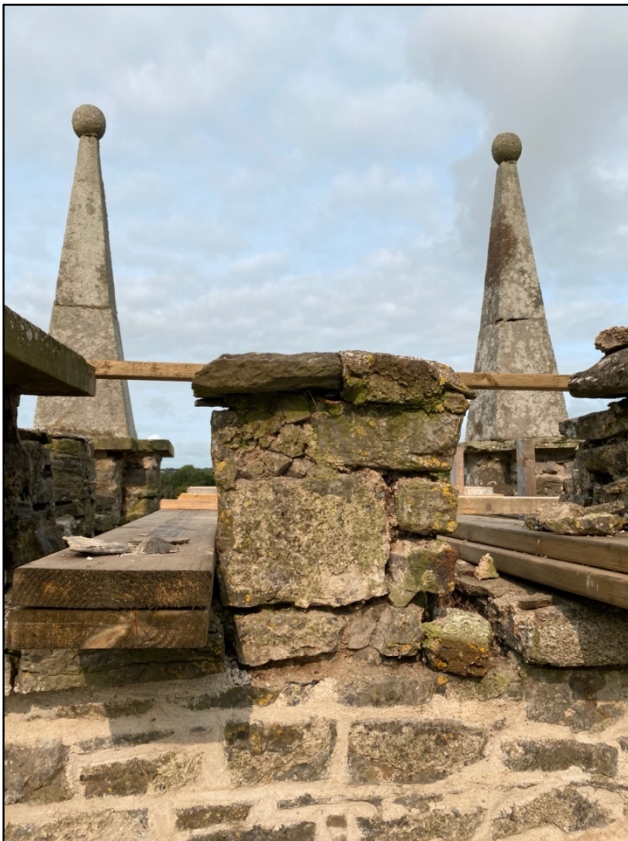
Plate 20: Condition of stone cappings and crenellations in advance of interventions.
