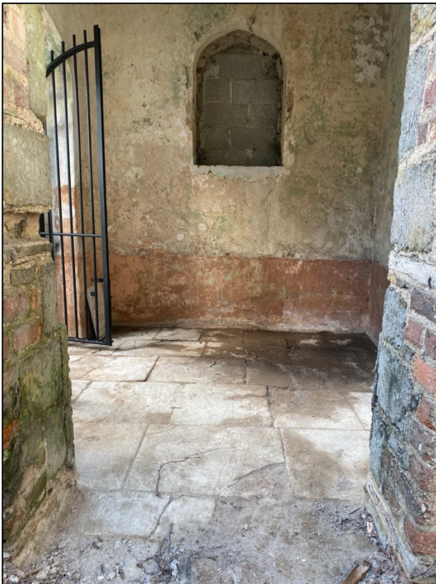
Plate 30: View of gate and cleared floor slabs in bell tower, facing west-northwest.
