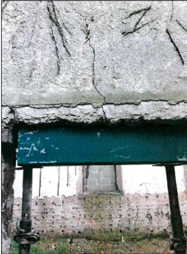
Plate 15: Vertical crack above door from vestry to nave.
