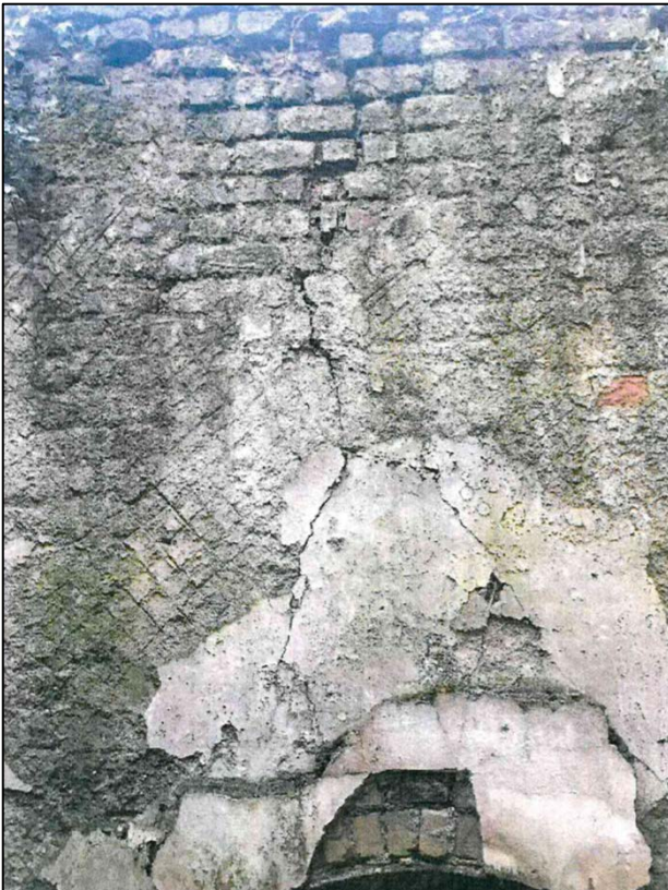
Plate 14: Crack above fireplace in vestry.
