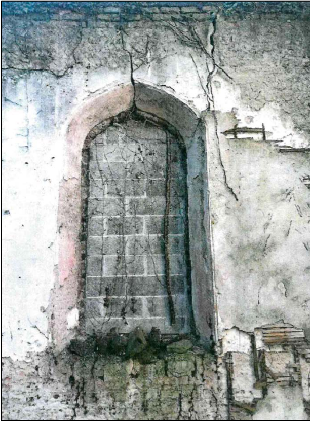
Plate 17: Cracking above window in south internal elevation.
