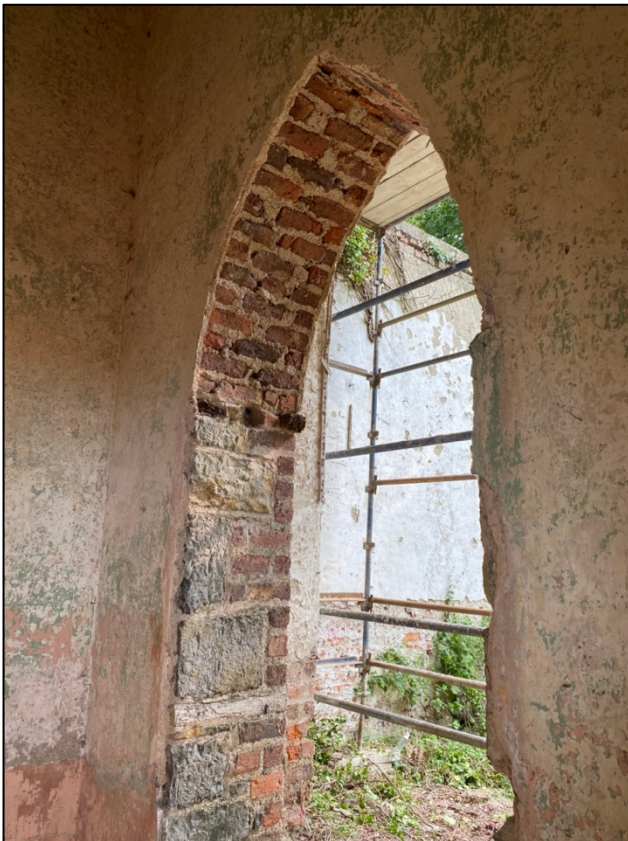
Plate 24: Detail of brickwork in door leading from bell tower to nave, facing northeast.
