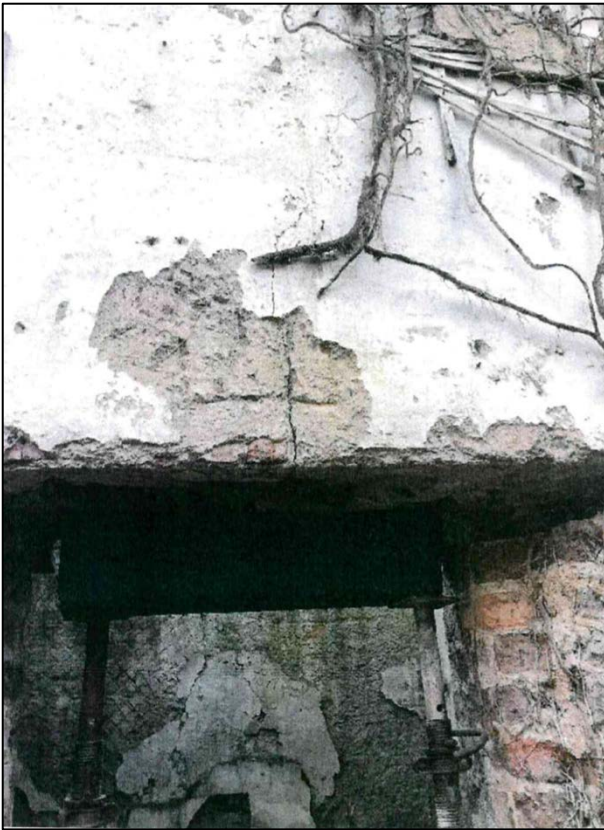
Plate 12: Vertical cracking above door opening to vestry at north internal elevation.
