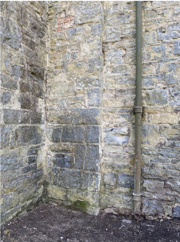
Plate 32: Repointing, and cast-iron water pipe on north elevation of bell tower, facing south-southwest.
