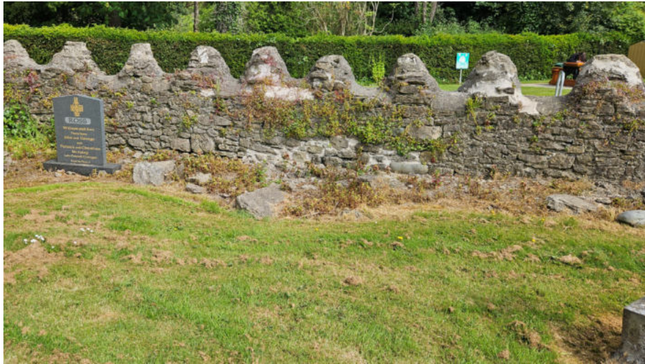
Plate 9: Vegetation growing on internal face of graveyard boundary wall from south
