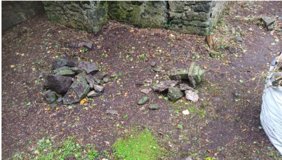
Plate 17: Loose stone collected and stored at southwestern side of boundary wall
