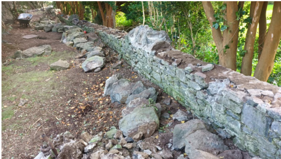
Plate 15: Coping stones stored along internal face of southern boundary wall from northwest
