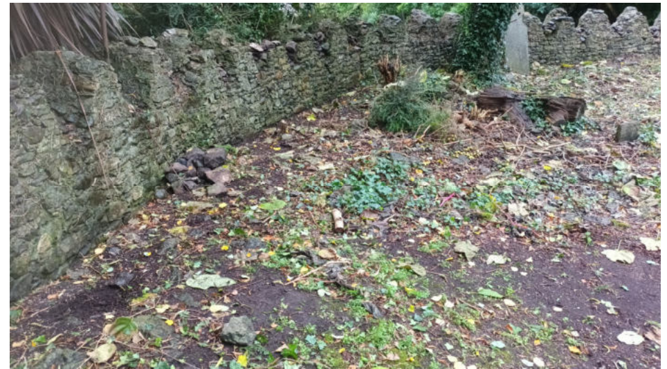
Plate 16: Loose stone collected and stored at southwestern side of boundary wall
