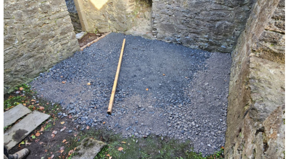
Plate 30: Crushed stone covering over floor level; residential tower; first floor; from south
