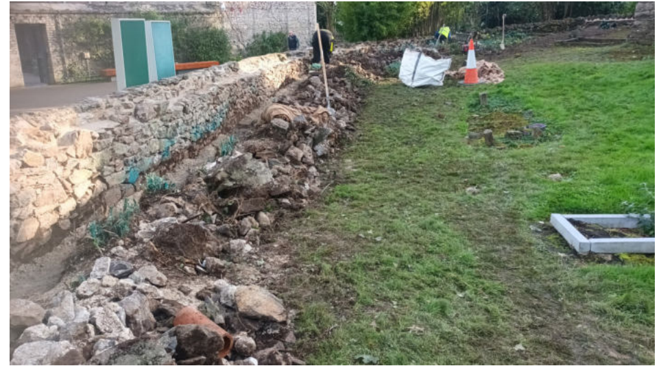
Plate 14: Loose stone retained at the internal side of boundary wall from northeast
