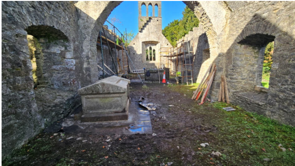
Plate 27: General view of church taken from the chancel with reconstructed tomb in foreground
