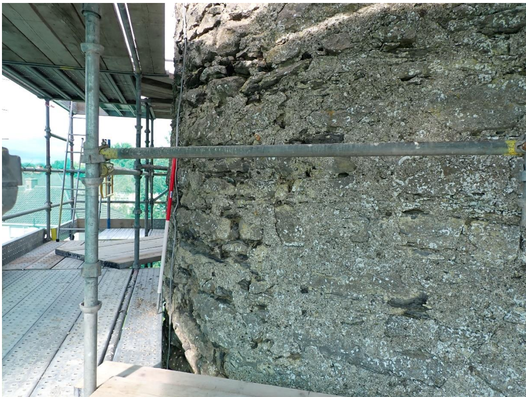
Plate 2: View looking west along the southeast side of the tower showing the effect of wind scour
