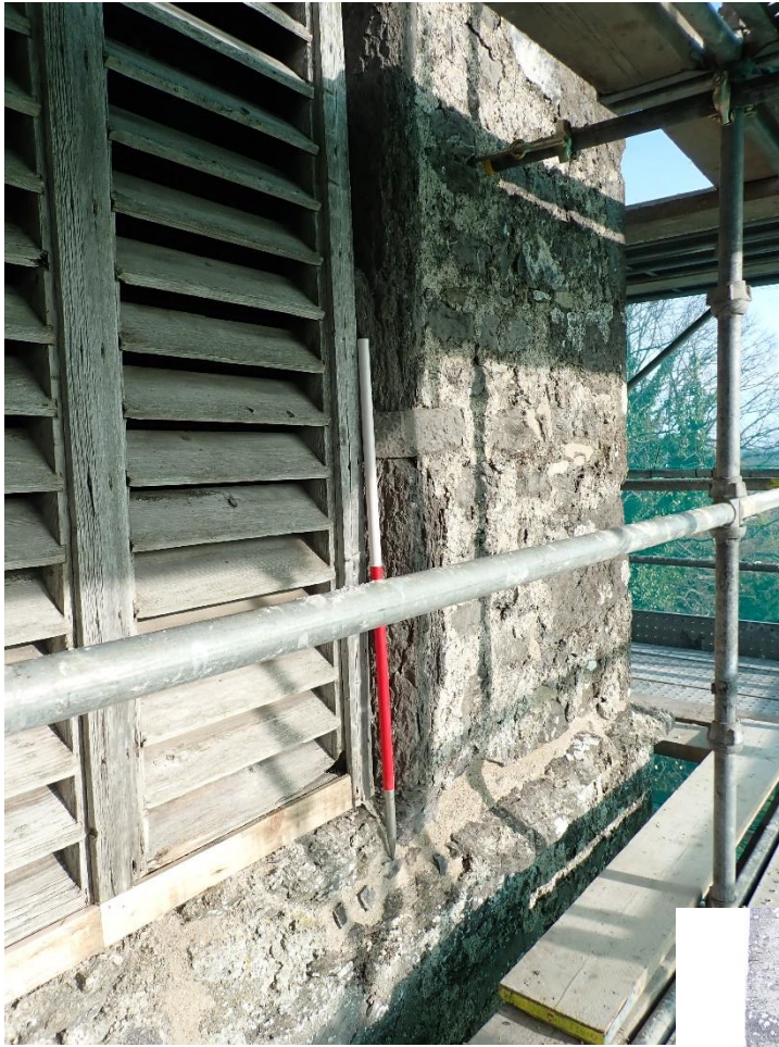
Plate 24: South side, replacement wooden sill and repointing of the string course at the base of the window.
