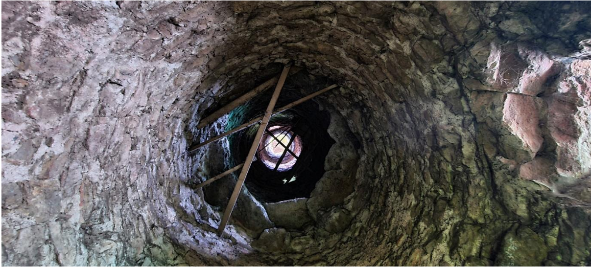
Plate 11: view looking up the tower from the basement; the inner lintels of the door are visible on the right and appear to be heat affected
