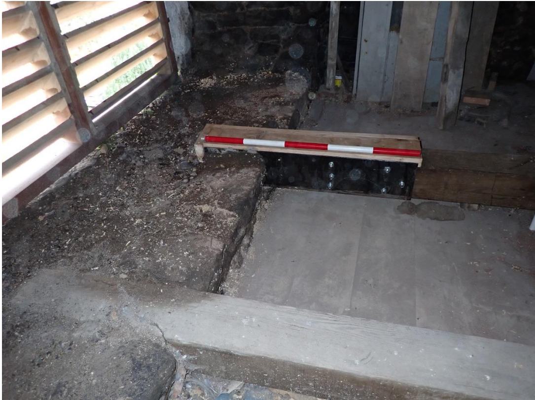
Plate 31: Interior, steel shoe in place to repair the end of one of the beams supporting the bell.
