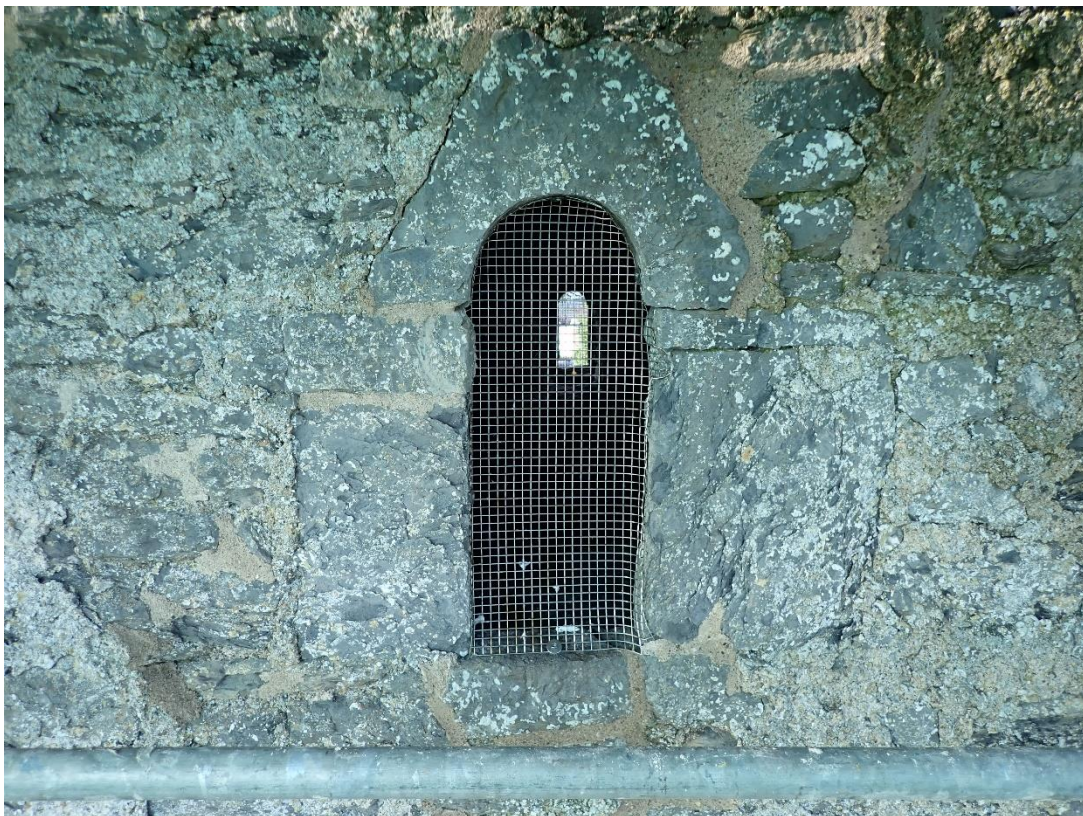
Plate 19: East face, round headed window with mesh grille inserted and re-pointing of surrounding stonework.
