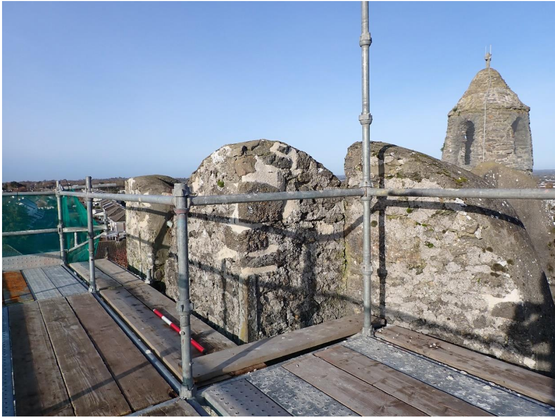
Plate 22: South face, re-pointing of the crenellations at the angle of the projecting stair tower.
