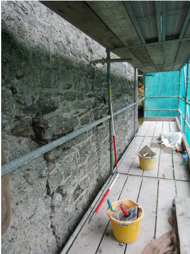
Plate 20: East face, crack at south side prior to repair.
