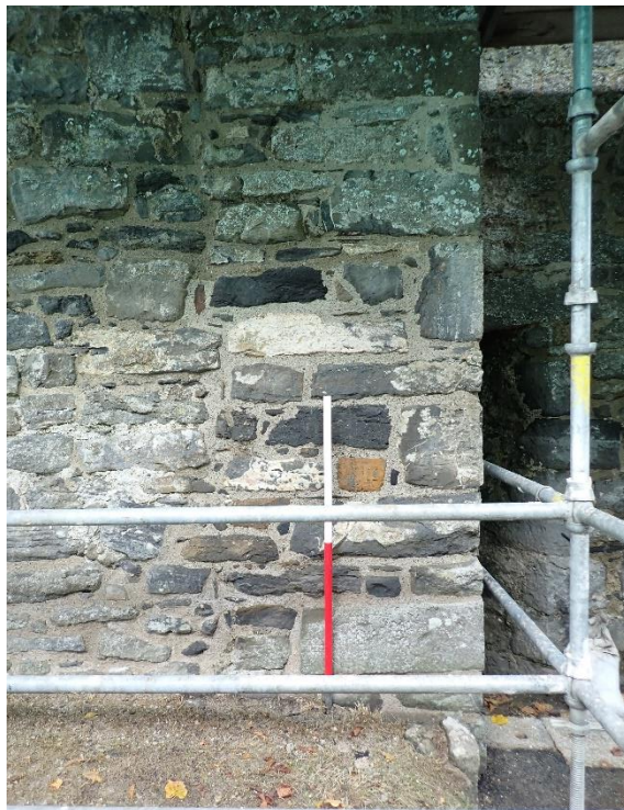
Plates 26-28: South side, repairs to the masonry join. Preparatory work, (Plate 26) followed by final pointing (Plate 27) and lower level, Plate 28.
