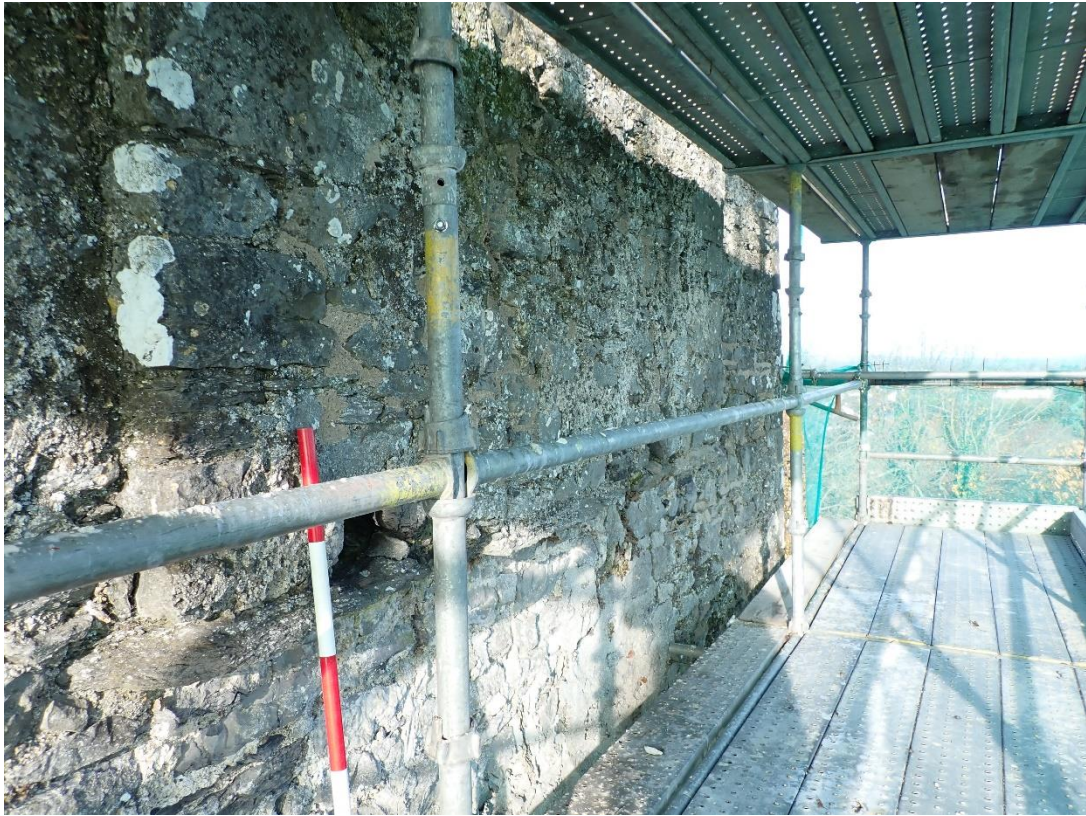
Plate 15: East face, base of projecting parapet, east face after vegetation removal and re-pointing
