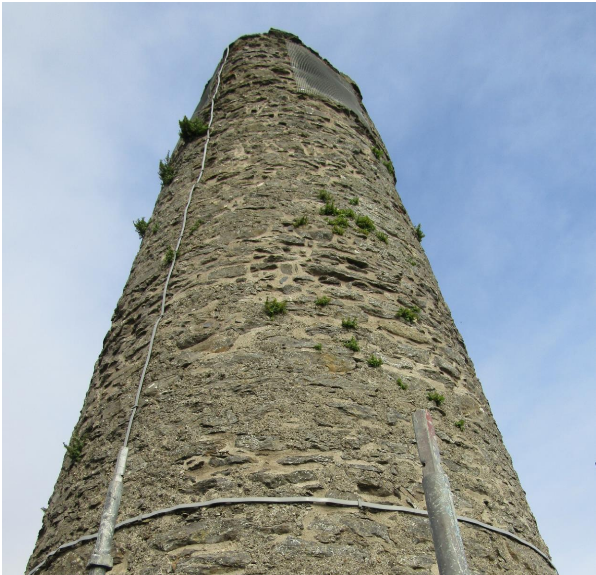
Plate 12: view looking NW at the upper floors of the tower showing some vegetation re-growth
