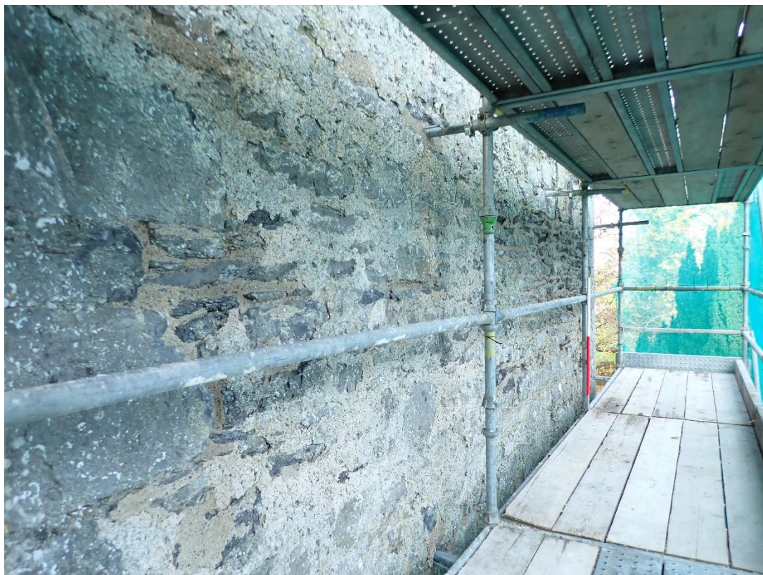
Plate 21: East face, crack at south end after repairs
