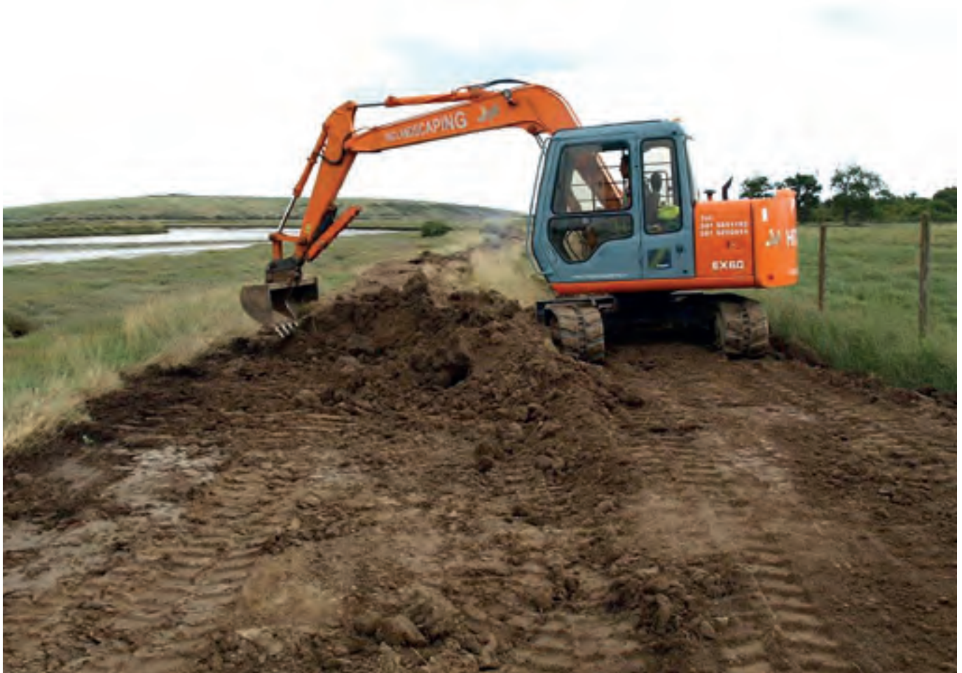
Figure 1: Flood embankment removal at the Rogerstown Estuary has restored the natural dynamics and flood storage capacity of the floodplain and increased the area of saltmarsh habitat.
