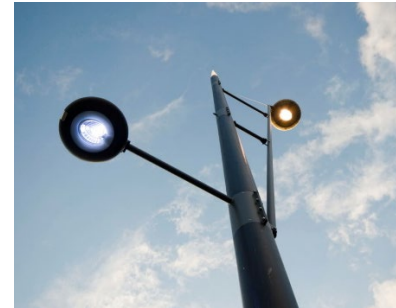
Twin Head Street Light (vehicle and pedestrian)
