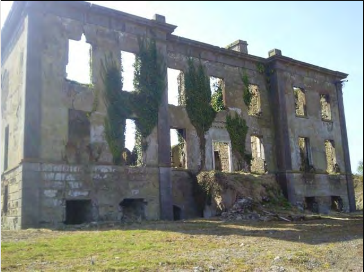
Plate 8: View of Westown house in ruins before restoration work was carried out.
