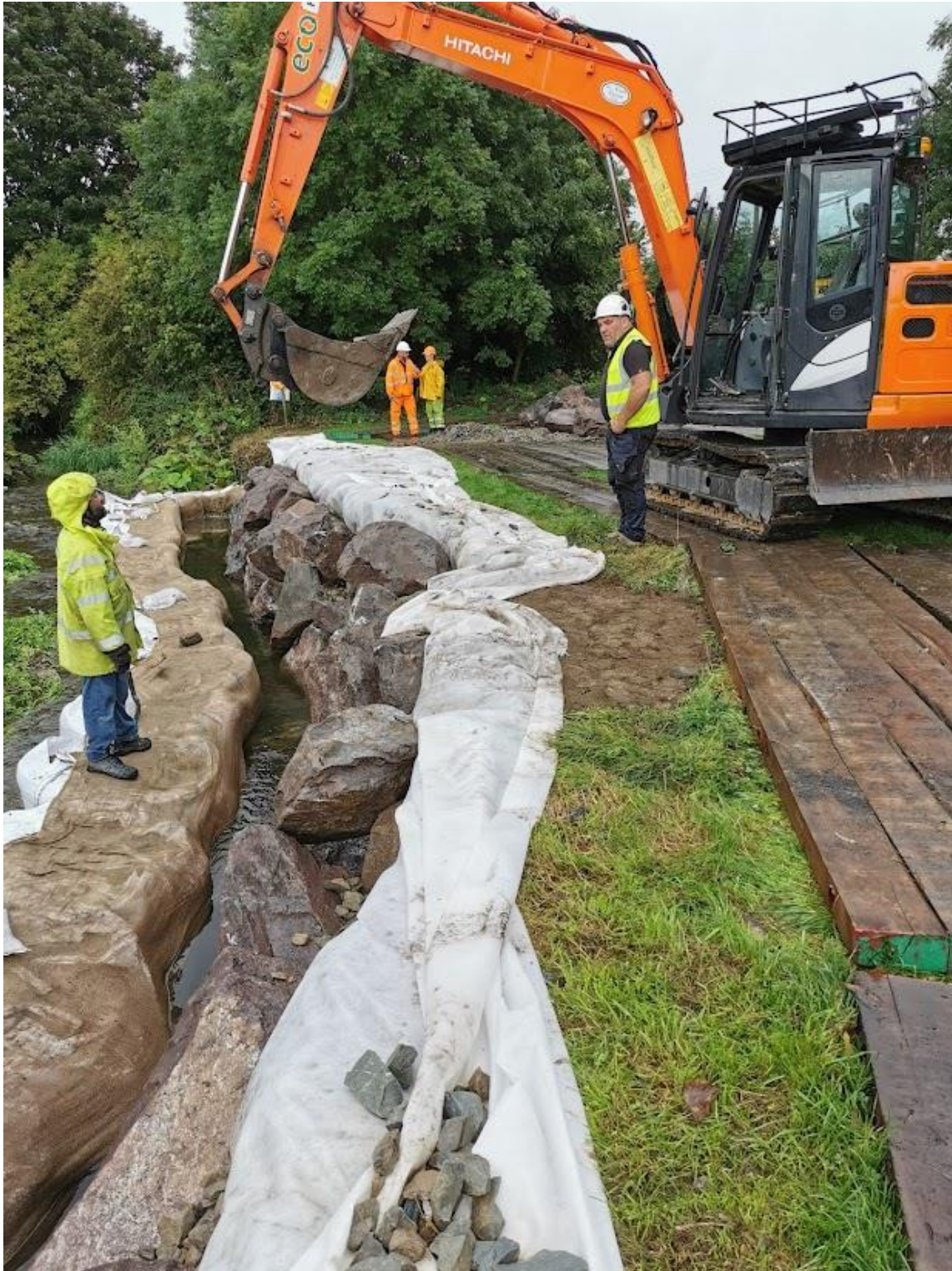
Plate 7: The area of the exposed burials has been infilled by soil and protected by rock armour
