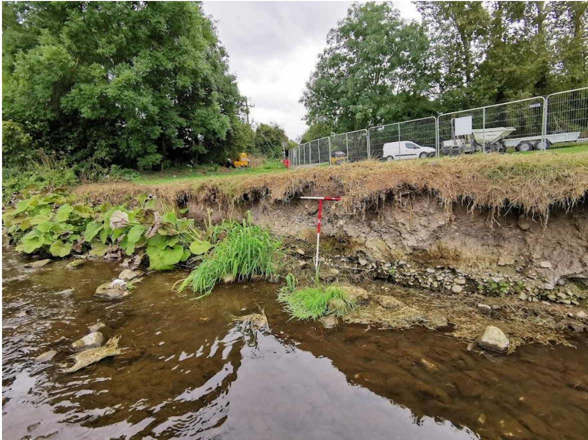
Plate 19: the east end of the section to be rock armoured, prior to the removal of vegetation. The bank appears to be decreasing marginally in height
