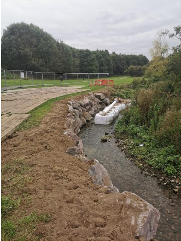
Plate 8: Looking west at soil capping of boulders, the sandbags are being removed
