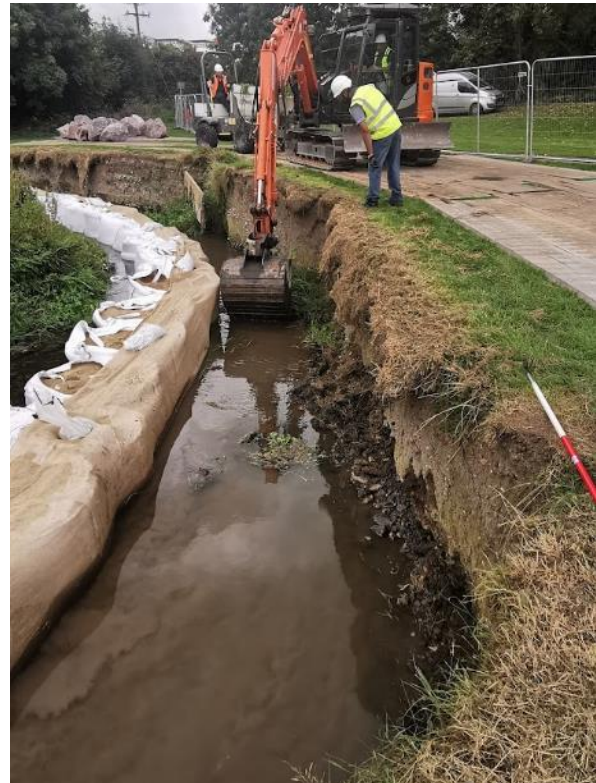
Plate 3: View looking east at cleaning operations, note bog mats on the surface.
