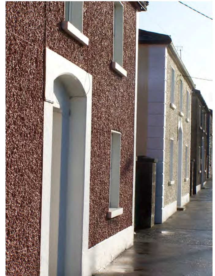
Above: Looking close up at the terrace of nineteenth century estate houses. They are kept in excellent condition and the variety of colour treatment is attractive. Treatment of surrounds to doors and windows suggests relatively recent replacement of render and introduction of quoins, the corner 'stones' applied to the middle house.
