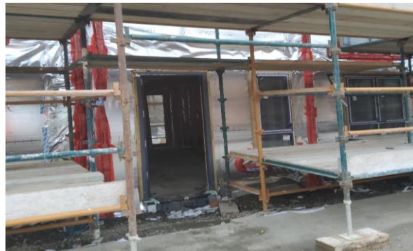
Timber frame dwelling in Dublin 15 with fire barrier (red) installed.
