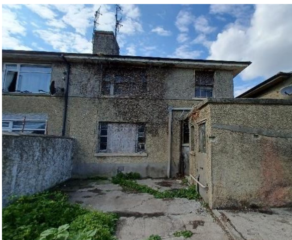
Derelict Property, 89 Portrane Ave., St Ita's Campus
