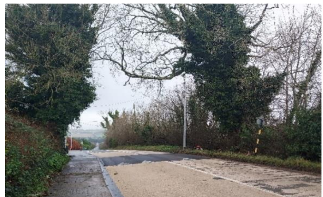
Naul- New Traffic Calming Ramps in the proximity of Naul National School
