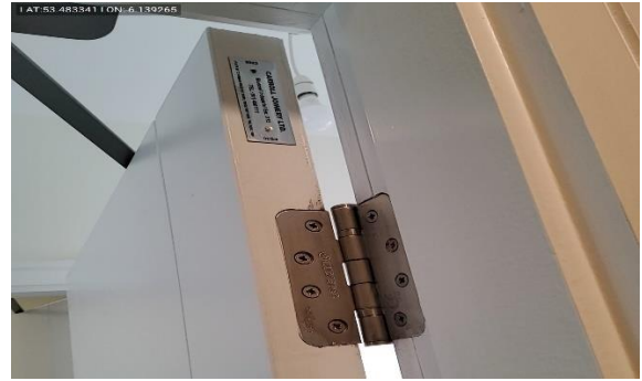
Checking hinges on a Fire Door in a 3 story dwelling house in Ballyboughal.
