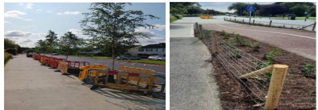
New tree and shrub planting along Brackenstown Road and St. Cronan's Avenue
