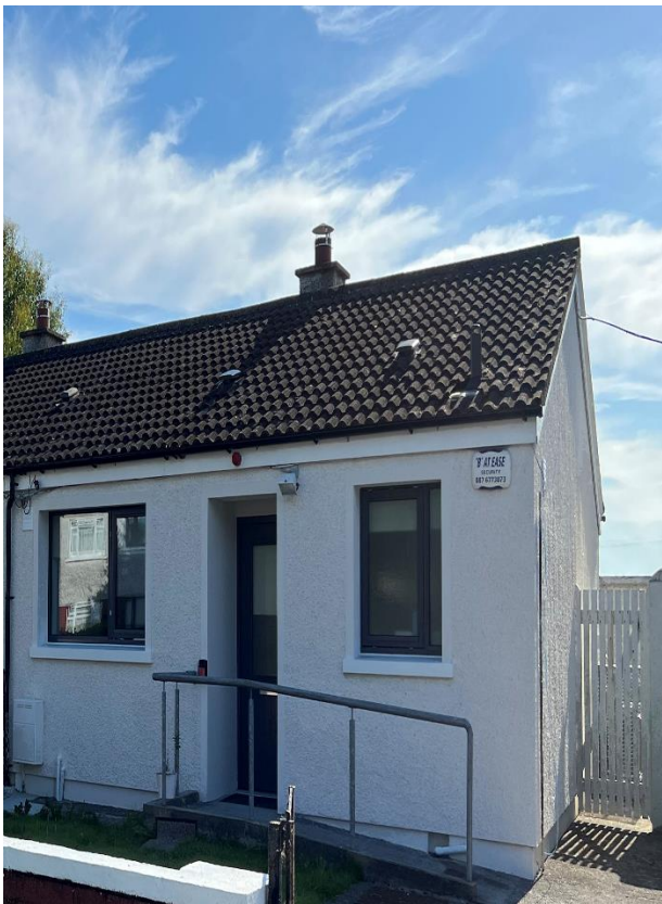
Post works – Strandmill Estate, Portmarnock (external wall insulation, new windows and doors)
