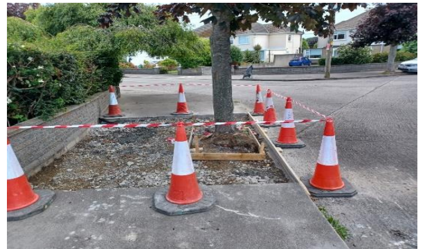
Broken Out Footpaths Stapolin Baldoyle
