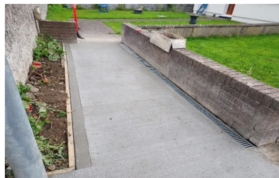
Footpath replacement works carried out in St. Paul's Crescent by Operations on behalf of Housing Department.
