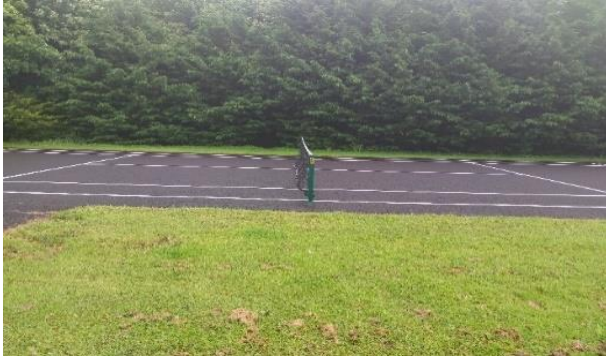
New tennis court built at the back open space in College Gate. Nets and posts placed on 17/7/2023.
