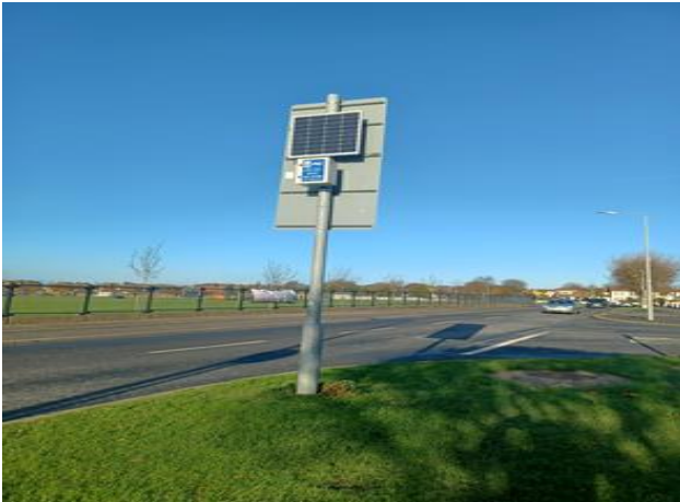
Conversion of electrical speed signal sign (by two) to Solar Power completed for Portmarnock Community School
