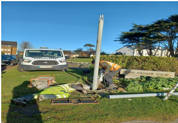
Traffic signal pole replaced due to rust at Binn Eadair View/Dublin Road junction
