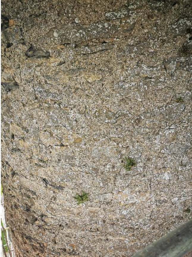
View of the south-east section of the tower prior to conservation with portion of possibly wind-scoured area at bottom left
