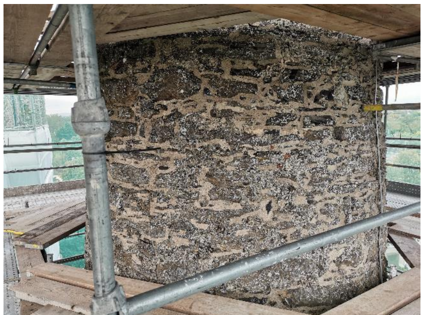
View of the fifth floor, exterior of the tower showing re-pointed joints. Note the presence of small pieces of brick within the existing render
