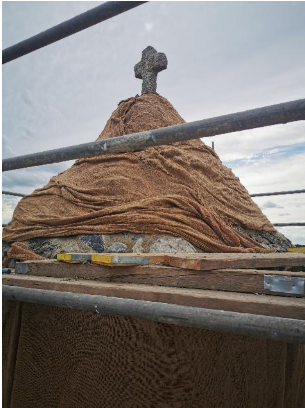
Roof with completed works covered in sacking; the cross has been stabilised
