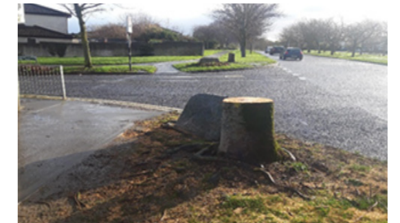
Removal of trees entering Kinsealy Court -Feltrim Road Junction to improve pedestrian/vehicular site lines. (Removal of stumps to follow with some footpath upgrades)
