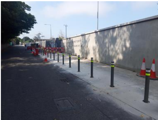
Installation of Bollards on Carrs Lane has commenced with the purpose of a 3m wide pedestrian walkway along the cemetery wall.
