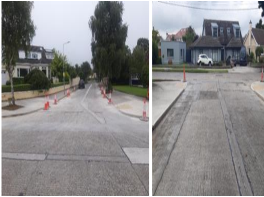
Two new Kerb Build outs with new tactile dishing in Offington – Howth.
