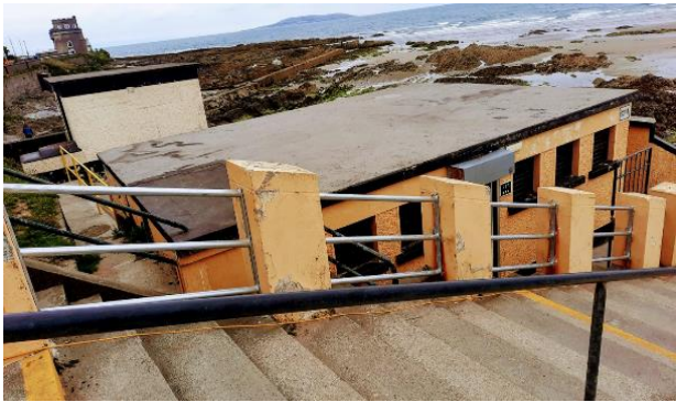
The rusted railings have been removed and new galvanised railings are being fitted at the steps to Velvet Strand from Portmarnock Promenade.
