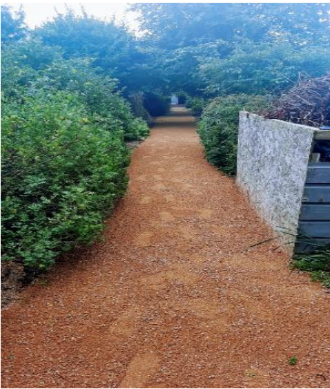
Pedestrian path resurfacing works as part of the current years works programme
