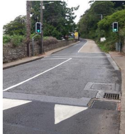
The pedestrian crossing at the bottom of Knockmaroon Hill has been relined
