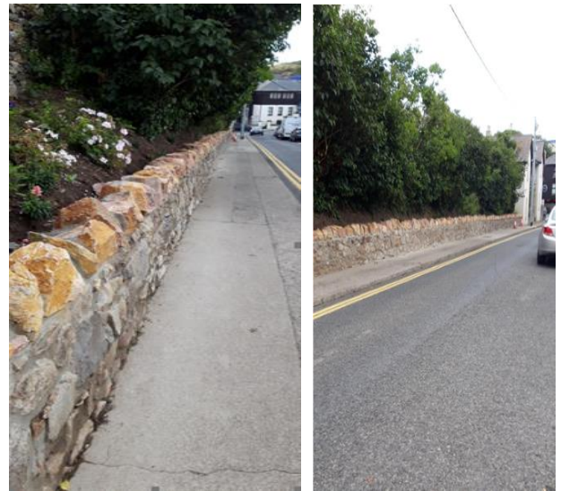
St Lawrence's Road retaining wall has been repaired and restored using a combination of existing stone and matching locally sourced stone. Over 50 meters of wall has, in sections, been rebuilt, repointed and had the capping restored.
