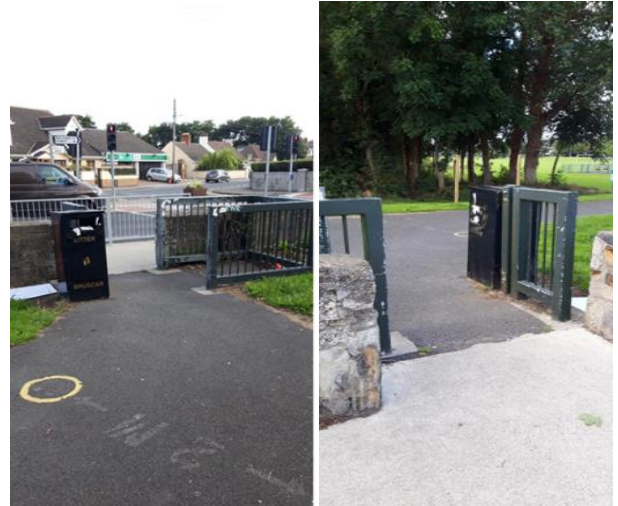
Provision of universal access into Seagrang Park from the R809 road was facilitated by the removal of the kissing gate and installation of a footpath barrier.
