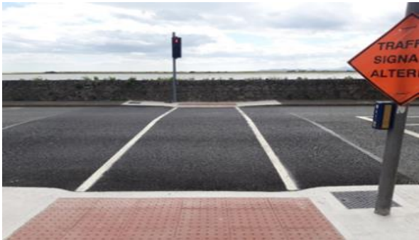
Upgraded pedestrian crossing and LED signals completed at Howth Road/Offington Park Junction
