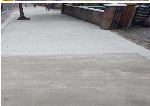
Footpath repair works with traffic management measures in place on Grange Road
