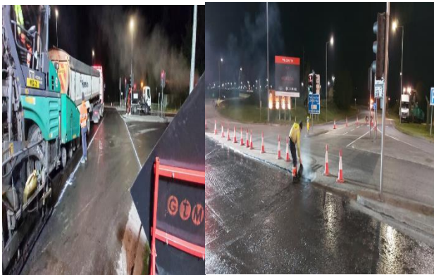
Pavement Works at Sillogue Essential application of seal to the road joint at Sillogue.
