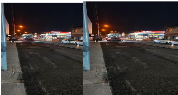
Application of the binder coat pre paving and rolling of the pavement following paving.
