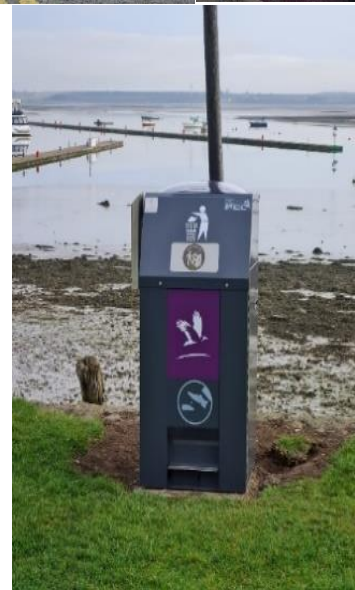
Delivery and Installation of 10 new Compactor Bins in the Howth Malahide area
