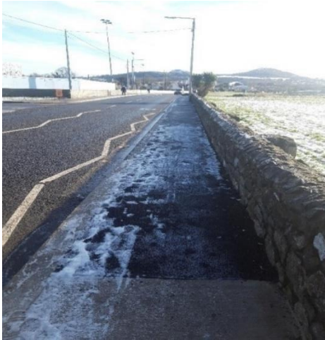
Section of footpath restored (Jan 21) in Bitumen by new signals (to be commissioned) on Greenfields Road Sutton by St Fintans Church.
