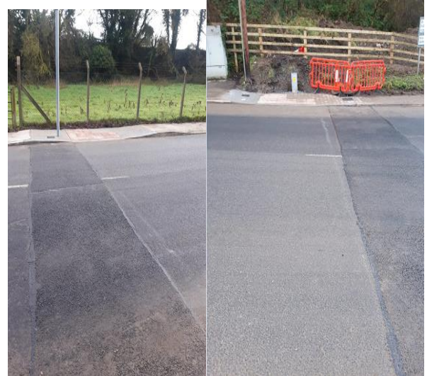
The Pedestrian Crossing in Naul Co. Dublin on the R108 at Naul GAA ground. Civil Works are now completed onsite. This was funded as part of the NTA Stimulus Plan
