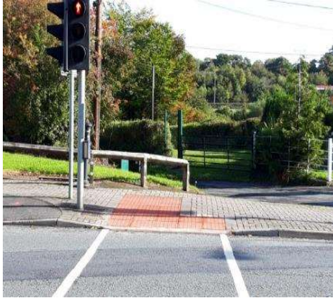
New tactile paving installed at Blanchardstown Main Street/Clonsilla Road junction completed in November.
