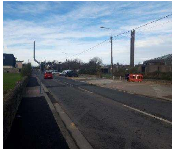
Civil works in progress near St Sabinas School- Greenfields Road, Sutton Including upgrade to footpath section
