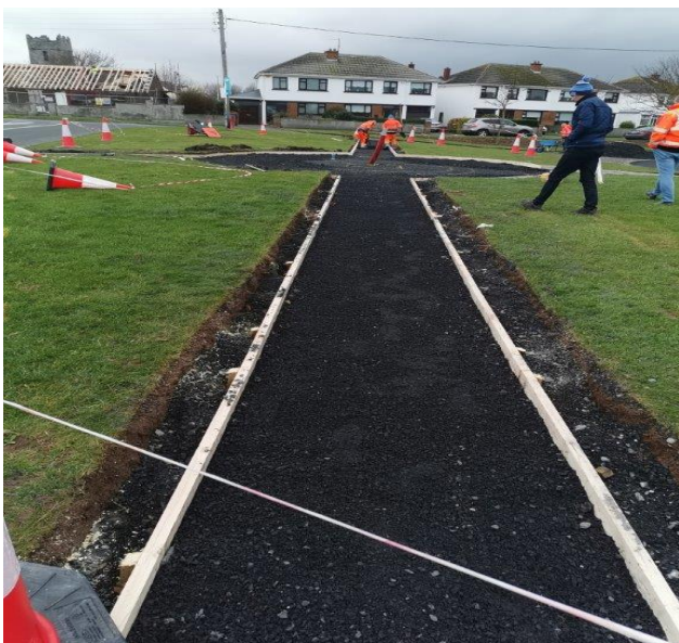
Swords Operations Staff carrying out preparatory works for Portrane Urban Village Renewal Scheme.
