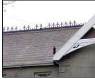
Fig. 10 Missing or damaged cresting
